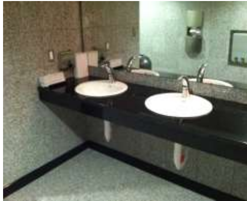
Example of accessible sink with knee and toe clearance, insulated pipes, and mirror with bottom edge at below 40" AFF.
