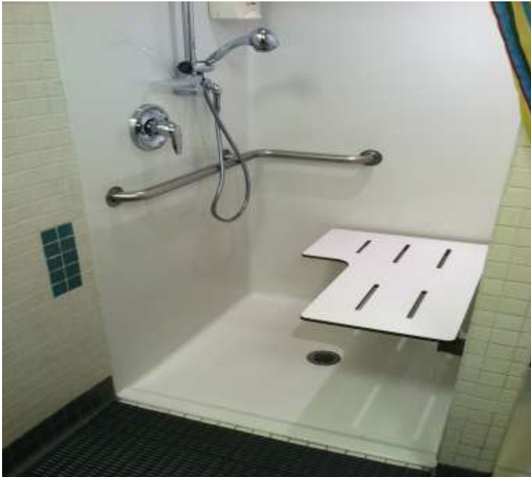
Example of an accessible transfer shower
