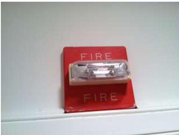
Example of built-in visual fire alarm.
